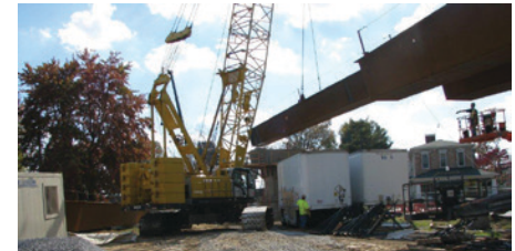
Operator David Harned and oiler Frank McDermott, on the Big 4 Walk Bridge in Jeffersonville, Indiana
