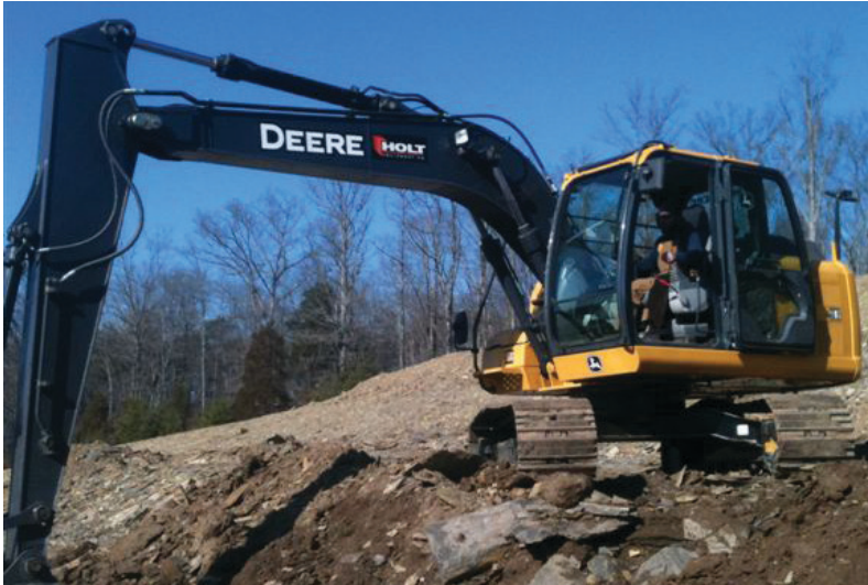
Boston Apprentice Nathaniel C. Parrish on the brand new John Deere 130 Excavator.
